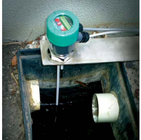
Sump pump control
