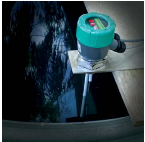
High level switch in water tank
