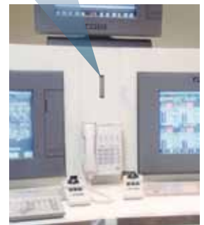
SIS Indicator in control room.
